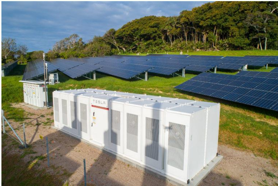
Lord Howe Island Microgrid
